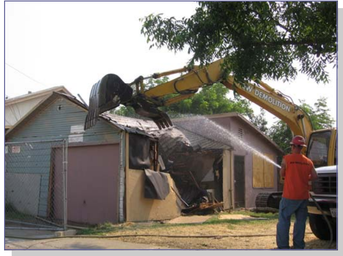
A bulldozer tears down the Wat Phou/George's Market on 14th Avenue in the Stockton Boulevard Redevelopment Area on July 10. SHRA plans to find a developer to build a single family home on the site.
